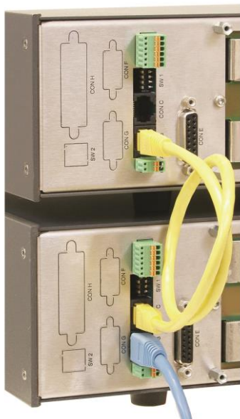
fig 4 - 22 Use standard UTP cables (RJ45) for Master / Slave operation.
